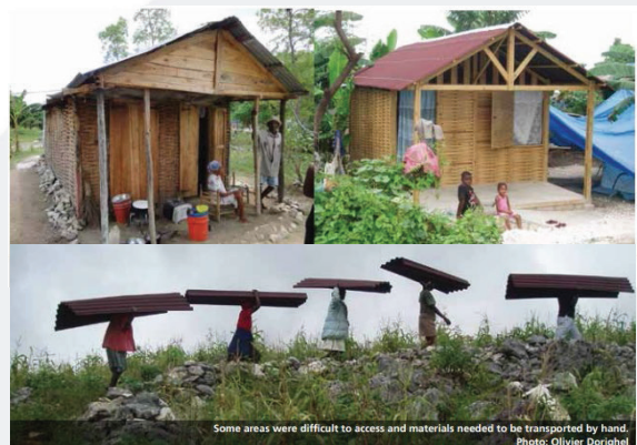
Some areas were difficult to access and materials needed to be transported by hand. Photo: Olivier Dorighel. No rights for pictures use.
